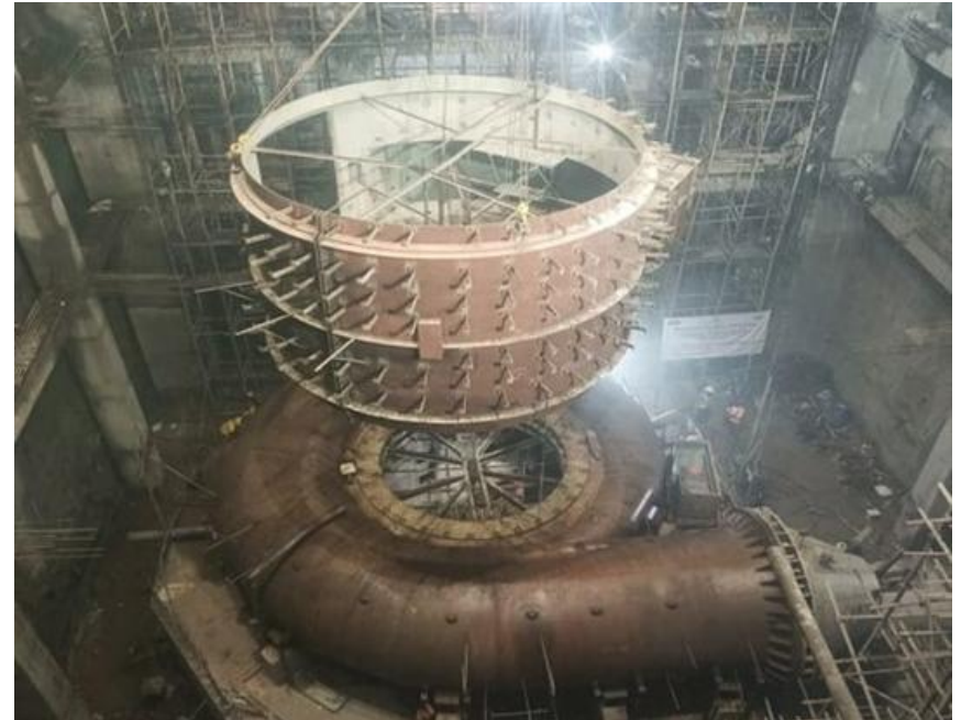
Machine Hall Unit 1 Spiral Casing
