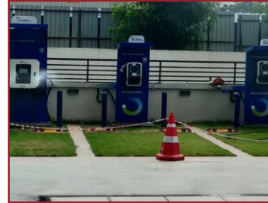
EV charging infra for employees
