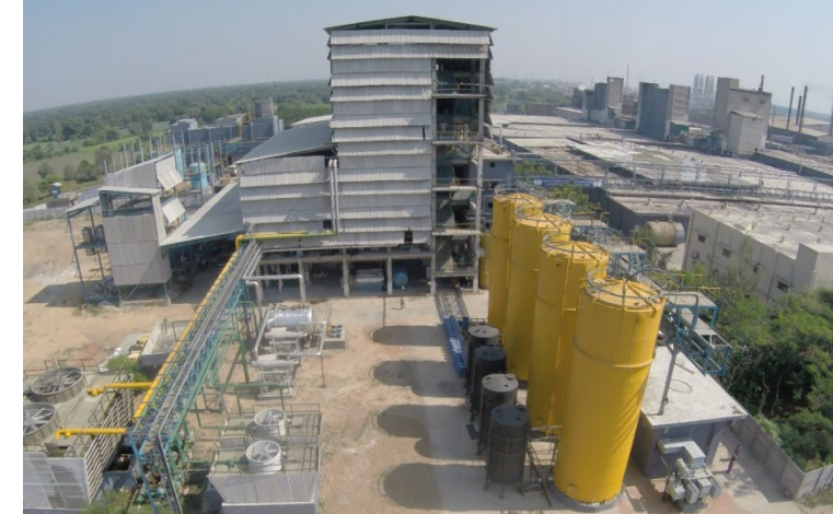
Multiple Effect Evaporator Plant (MEEP)
