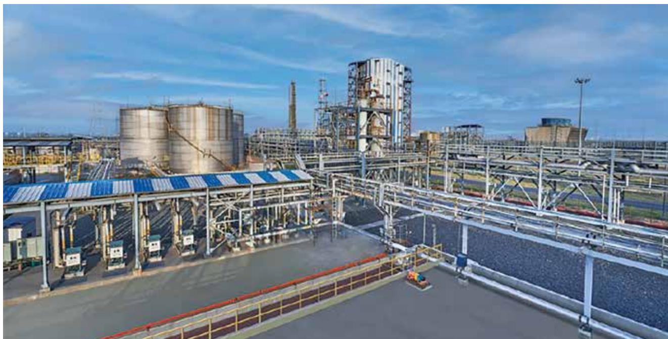
Dahej Nitric Acid Complex
