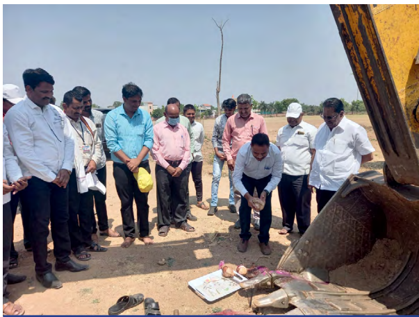
Desilting and widening of a percolation tank at Yashwant Rao Mahavidyalaya, Karmala, Solapur Maharashtra
