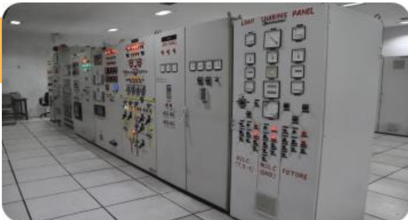
Cogeneration control panel
