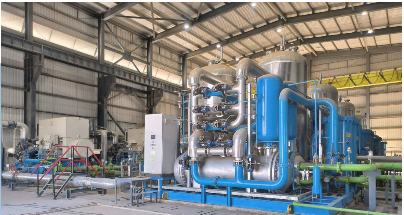
Compressed air station at Kutch Copper Limited, Gujarat
