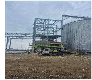
Ethanol plant, Jammu
