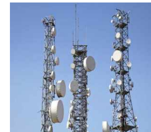
5G Telecom Towers
