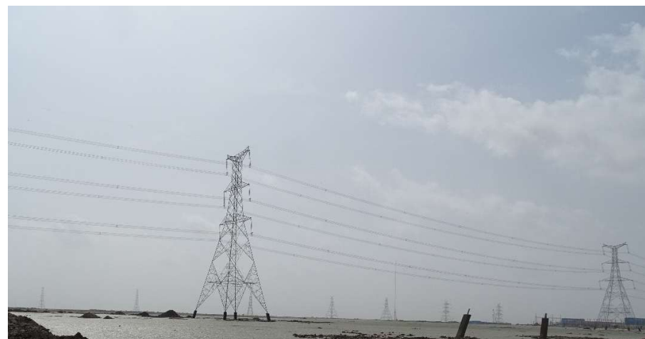
765 kV D/C Transmission lines in Khavda
