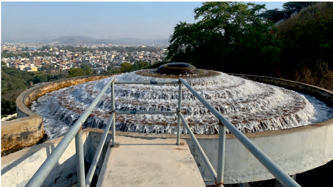
Waste Water Treatment Plant, AMRUT Scheme, Udaipur, Rajasthan
