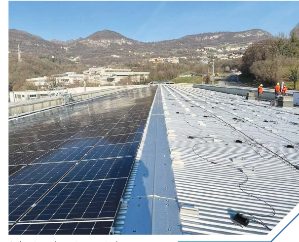
Solar Panels at Bione, Italy
