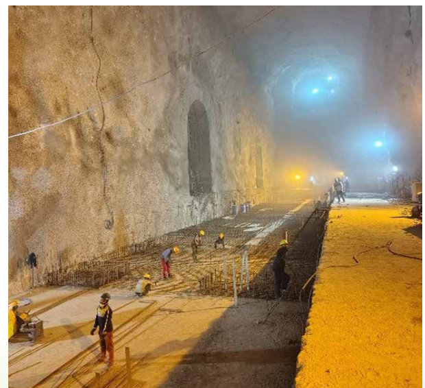
TRANSFORMER CAVERN – 850 MW RATLE PROJECT (UT OF J&K)
