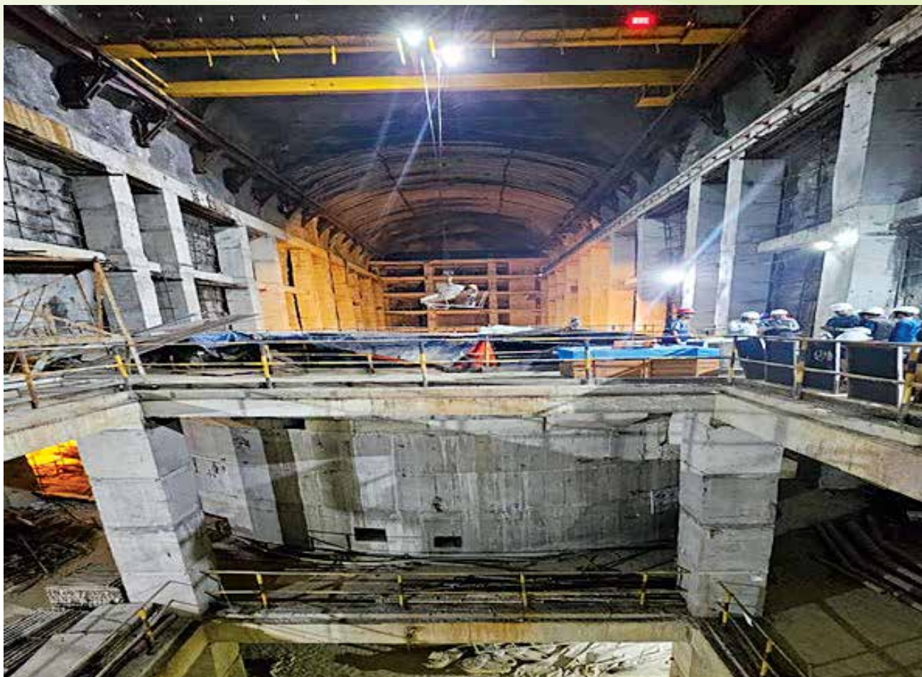
POWER HOUSE – 500 MW TEESTA-VI PROJECT (SIKKIM)
