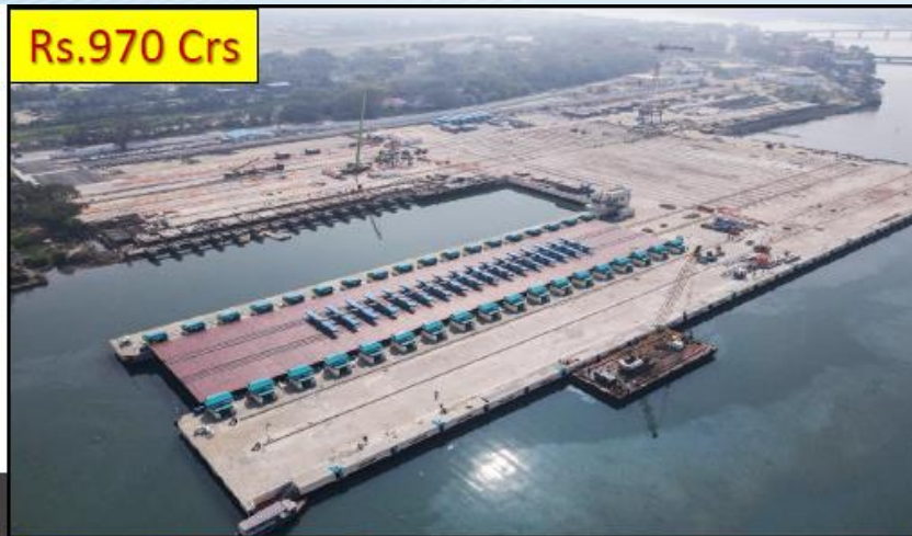
International Ship Repair Facility – with 6000 T Shiplift
