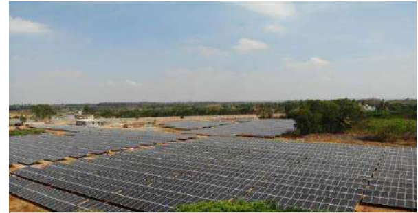
Solar Panels at HRGRDC, Bengaluru
