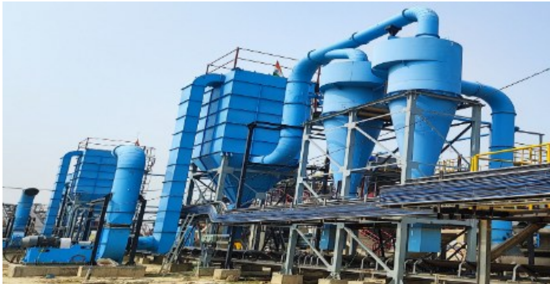
CBG Plant at Budaun- Milling Section
