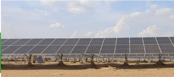
2012 MWp Ground Mounted project at Bikaner, Rajasthan
