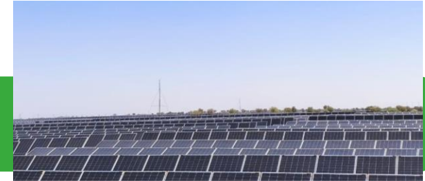
412.5 MWp Ground Mounted project at Bikaner, Rajasthan
