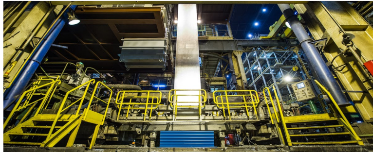
Continuous galvanizing line for cold rolling mills
