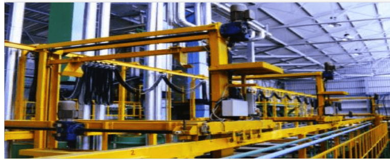
Power handling system for paint shopfloor
