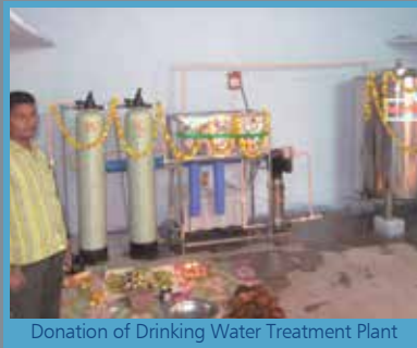
Donation of Drinking Water Treatment Plant
