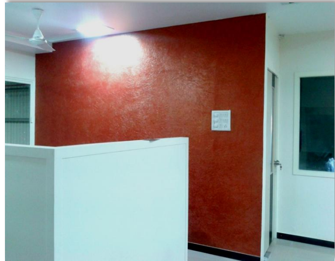
Wall Paneling - (V-Board)
