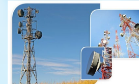
Microwave Radio Backhaul Solution
