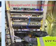
Fiber Optic Transmission System - FOTS
