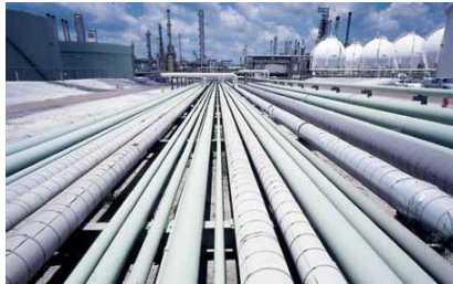
Anti Corrosive Material
