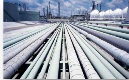
Anti Corrosive Material
