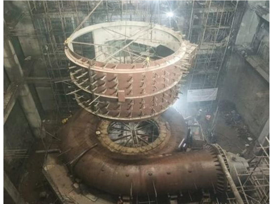
Machine Hall Unit 1 Spiral Casing
