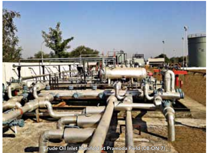
Crude Oil Inlet Manifold at Pramoda Field (CB-ON-7)
