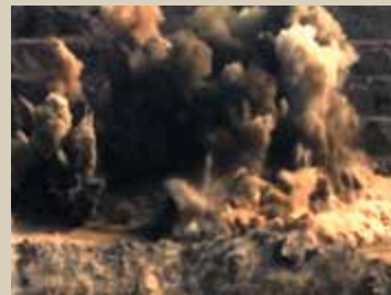
Successful firing with combined production and trim blast at Rampura open cast
