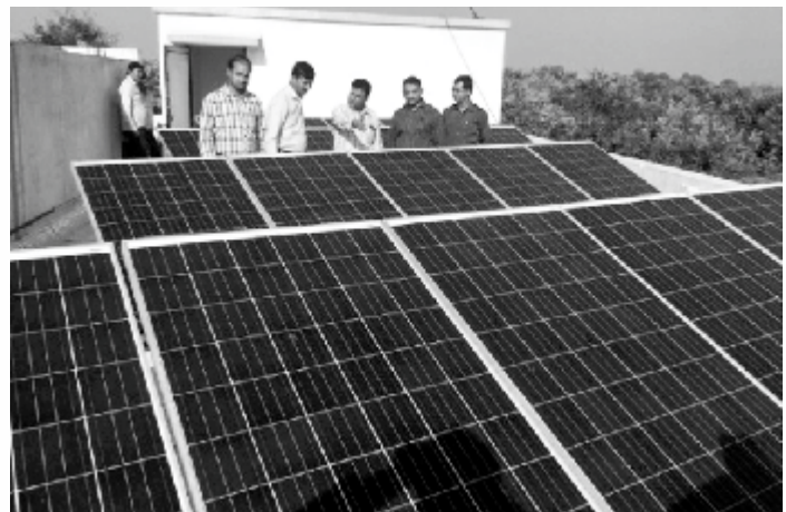
Solar panel at CNG station
