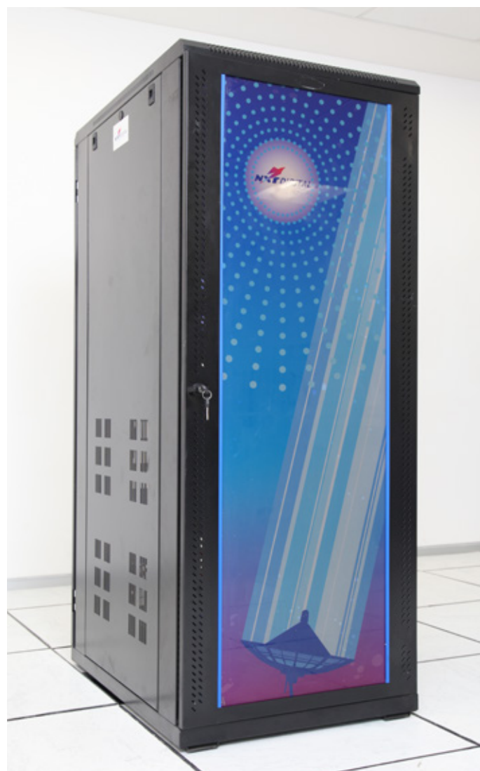
COPE (Cable Operator Premises Equipment)
