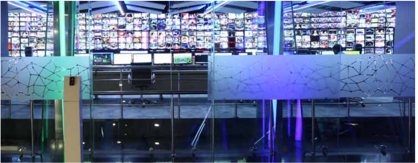
State-of-the-art Broadcast Facility at Noida
