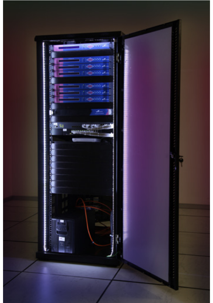
COPE (Cable Operator Premises Equipment)
