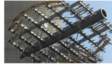
Spray Headers for Flue Gas desulphurization
