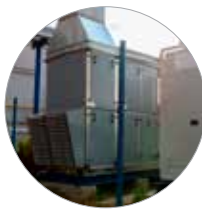
Air handling units
