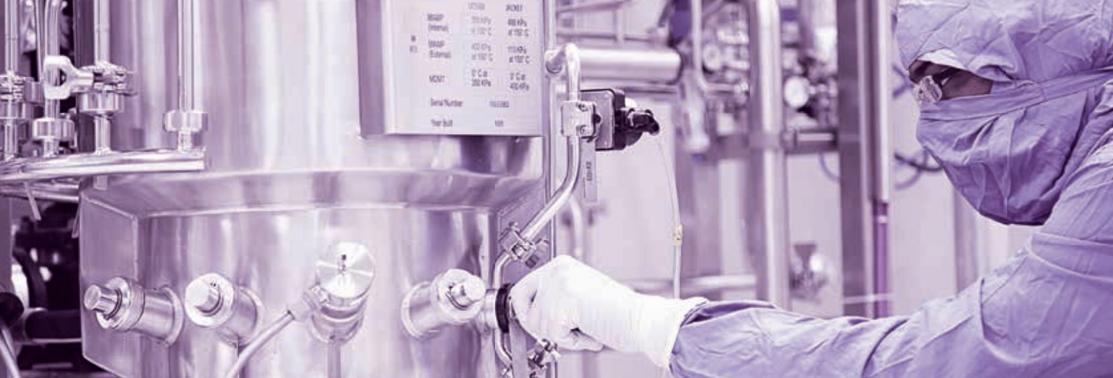
Lupinytt at Biotech manufacturing facility, Pune, India
