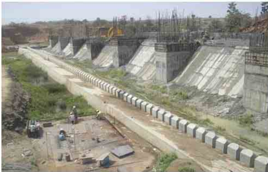
JACK WELL CUM PUMP HOUSE - MIHAN
