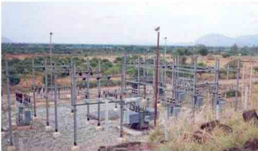
Project: Southern Power District Co of AP, Tirupati, AP.
