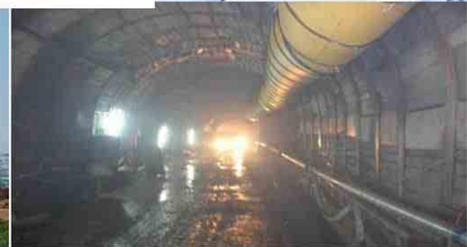
Project: Duhagan Hydro Electric Project Scope: Upstream Head Race Tunnel – Tunnel inside view
