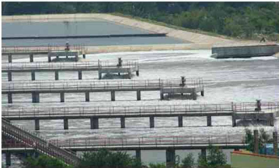
FACCATATIVE AERATED LAGOONS-339MLD STP AMBERPET, HYDERABAD
