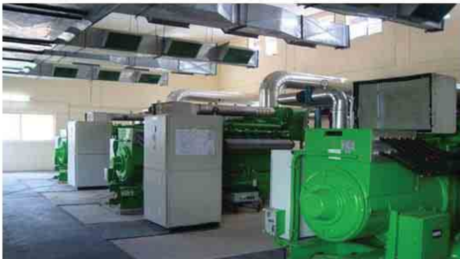
STP BIO GAS GENERATORS -339MLD STP AMBERPET
