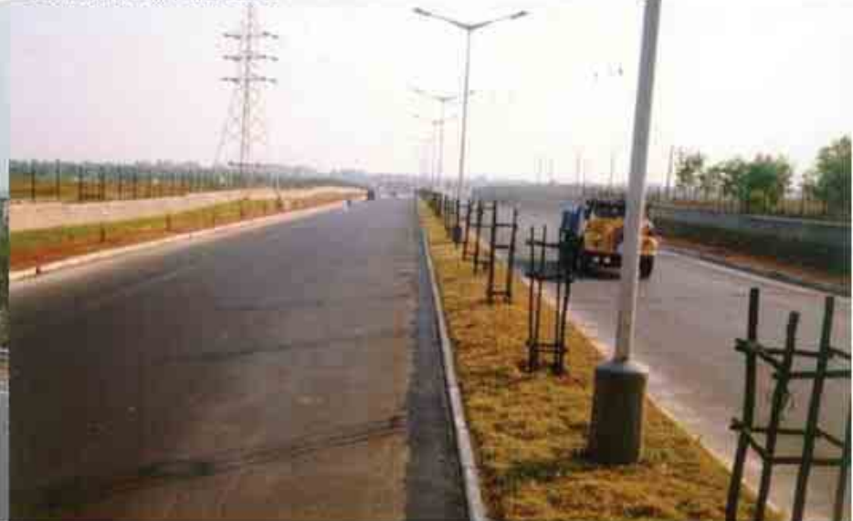
Project: Construction of carriageway of ring road along with cross drainage works in Bangalore city
