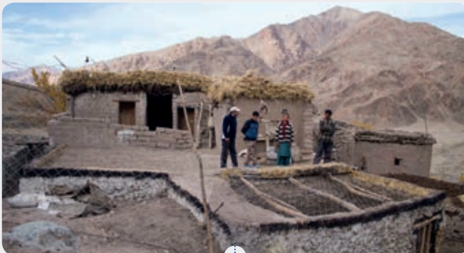
Construction of corrals for the communities to safeguard their livestock; Photo credit – Dawa Tsering WWF India
