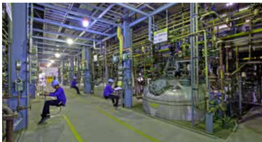
Multi-product plant in Jambusar
