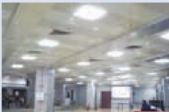
'Signature Series' LED tiles meeting the high lighting performance with aesthetics of the Airport Authorities
