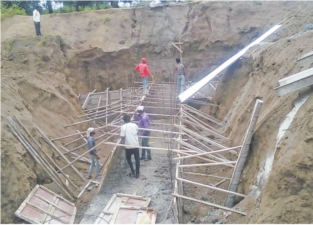
Construction of cement nala bund in the drought-prone area of Jalna, Maharashtra
