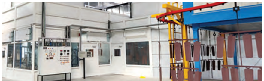
▲ Auto Powder coating at Swiss make plant installed at Kundaim Plant
