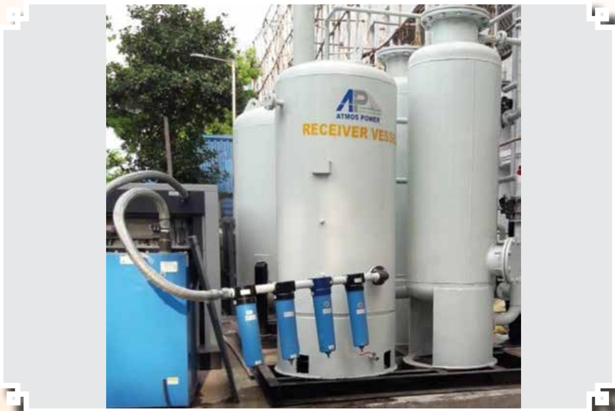
RCF installed PSA based Oxygen Generator Unit at Shatabdi Hospital, Mumbai under CSR Scheme
