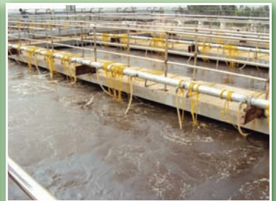
ZLD - Biological Plant
