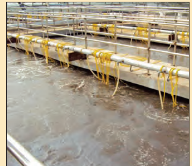
ZLD - Biological Plant
