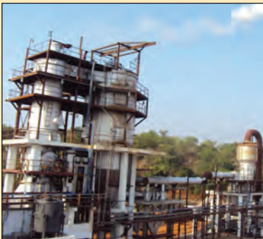
Zero Liquid Discharge (ZLD) unit at Srikakulam Biological Plant
