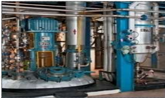
Agro Chemical Plant Panoli
