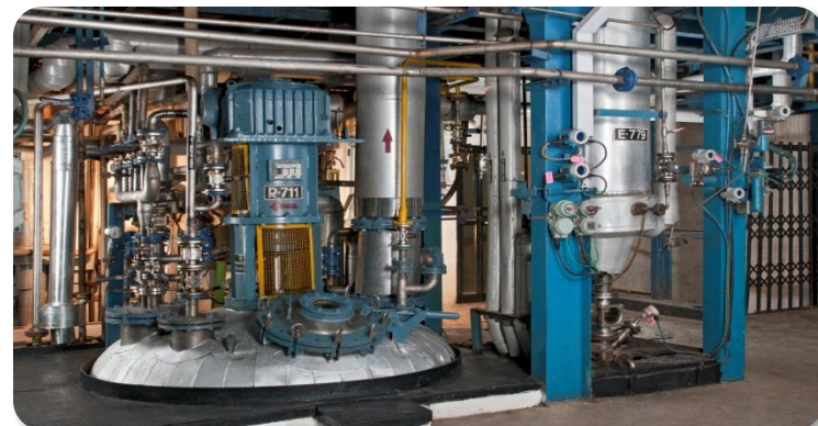
Agro Chemical Plant - Panoli
