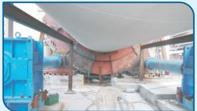
Hot Air Recirculation in line-1 IKN cooler installed as part of the Company's Power Saving Initiative
