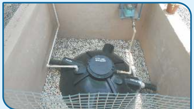
Sewage Treatment Plant installed at the Kalol grinding unit is a step towards water conservation
