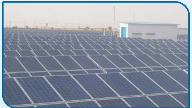
6 MW Solar Power Plant installed at Jodhpur as part of the Company's commitment towards a sustainable environment
