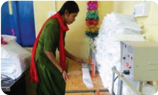
Installed sanitary napkin making machine and organized awareness program near Durg plant
