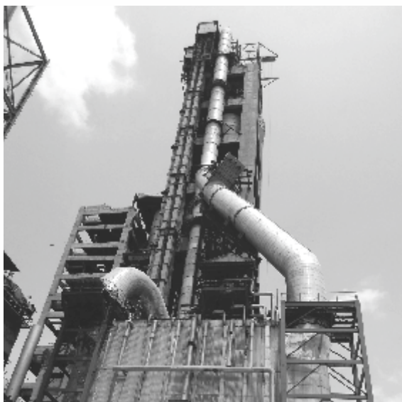
Hybrid ESP with integrated bag house for efficient emission control.
