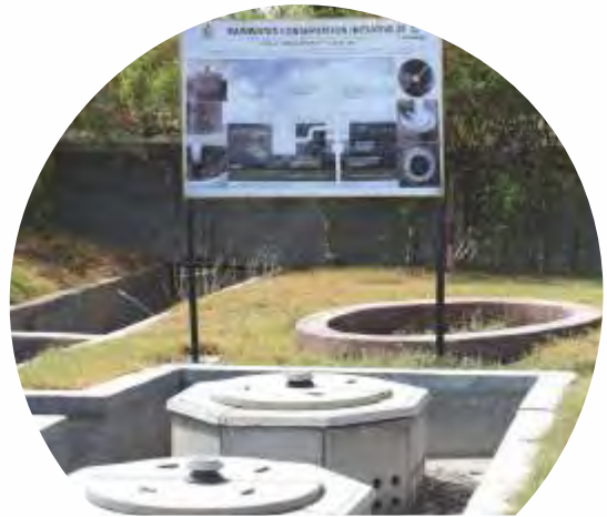
RAINWATER HARVESTING AT KALOL PLANT
