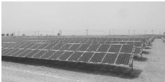
6 MW Solar Power Plant at Phalodi, Rajasthan
