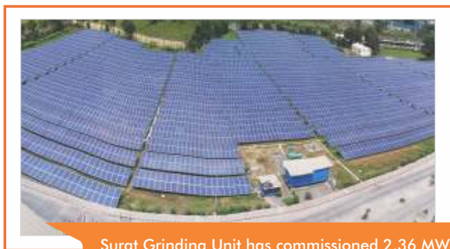
Surat Grinding Unit has commissioned 2.36 MW captive solar power plant that meets about 12 % of the total power requirement of the Unit
