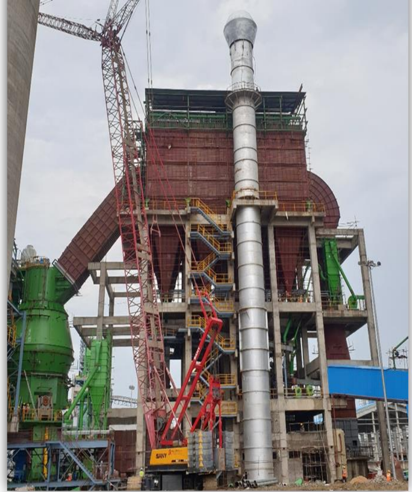
Cement Mill Bag House
