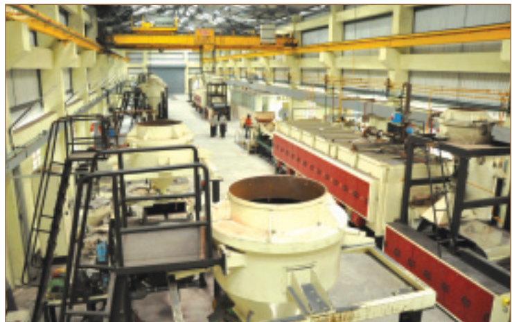
Sponge Iron Powder Plant at R&D Centre, Hyderabad
