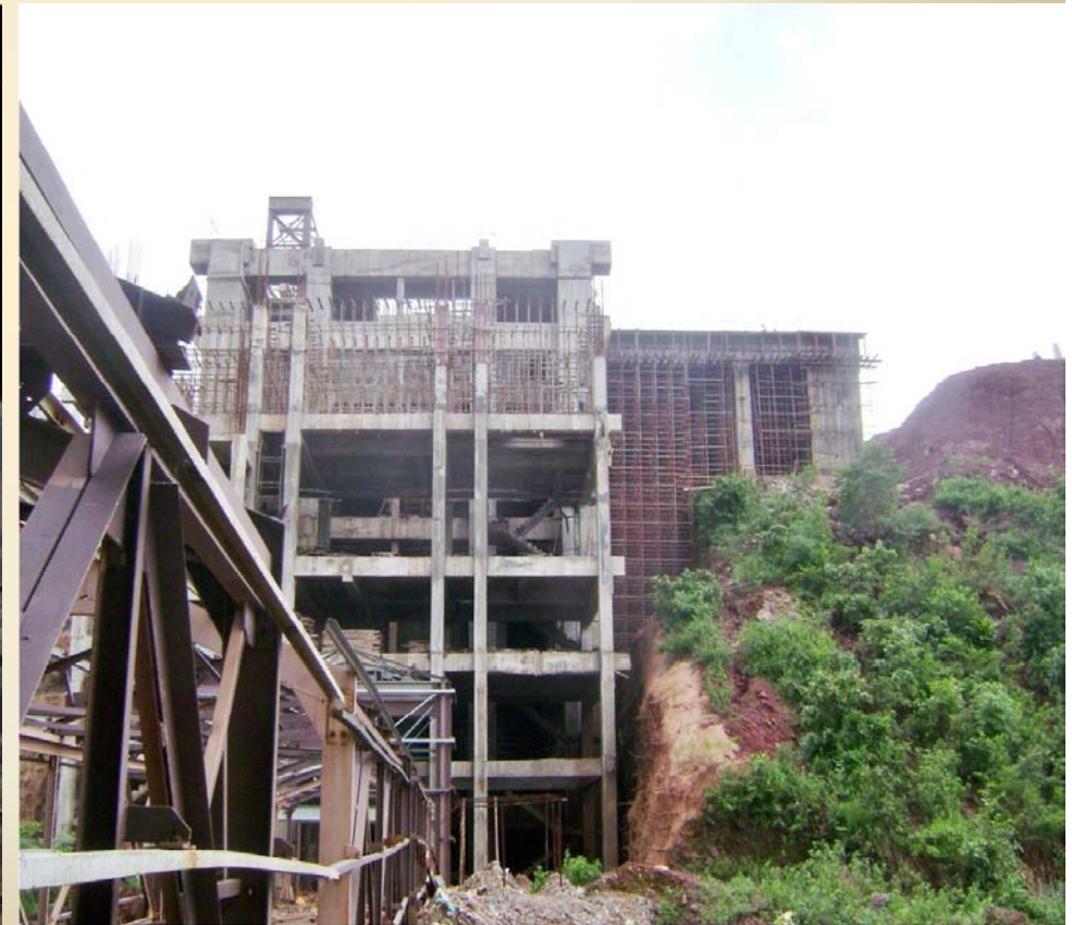
PCH EOB DP Conveyor
