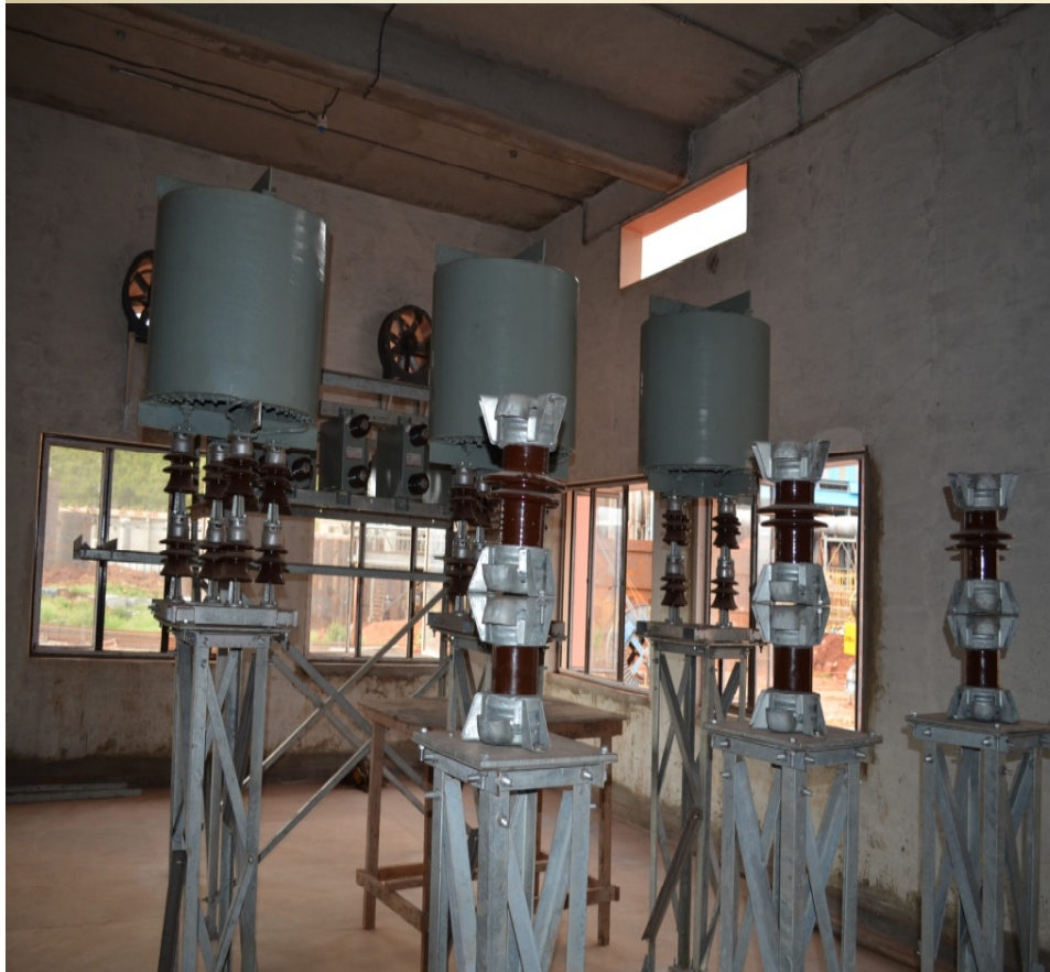
MRSS Capacitor Room
